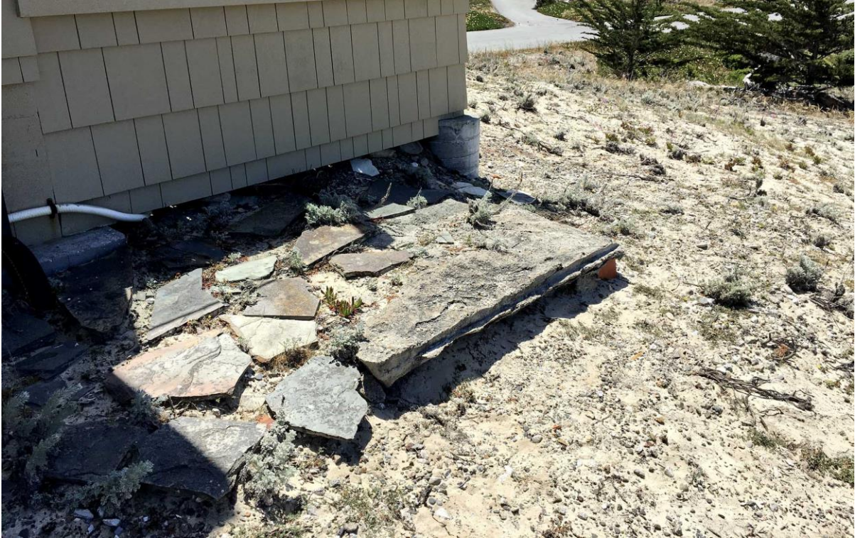
Photo 9. Remnant of concrete walkway on southwest corner of deck. Should be removed.
